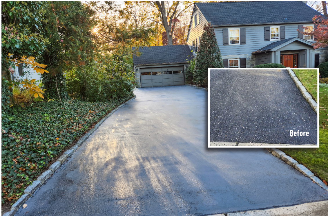
Powder pigment was added to the Surface Armor™ to achieve a similar finish to the original asphalt. The 1250 ft 2 driveway was completely resurfaced in approximately 5 hours.
