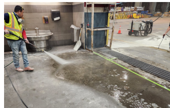
Area to be repaired is washed and all loose material is removed.
