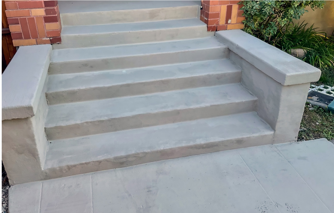
Restoration complete in 5 hours using one bag of Elephant Armor® DOT and one bag of Surface Armor™ without the need for the traditional and extremely costly, time consuming deconstruction/reconstruction process greatly extending its life-cycle.
