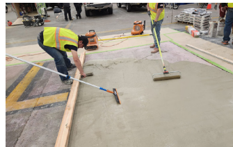
Elephant Armor® is easily placed and levelled with GST Rollers and Squeegee Trowels.
