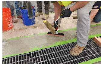
The second damaged area on the outside perimeter of drain is now overlaid with Elephant Armor®.
