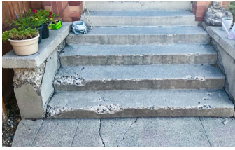
Severely spalled and degraded stairway, properly cleaned and sealed with Ecobeton® Vetrofluid®
