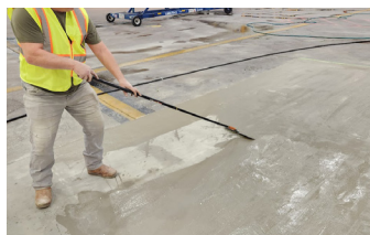
A coat of Surface Armor® is applied over the entire repaired (filled) area.
