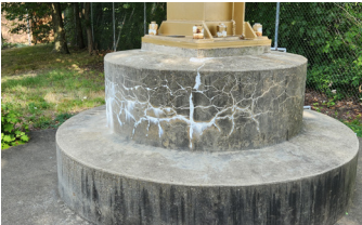
Ageing concrete showing cracking and calcium being released and formation of mold due to water retention.
