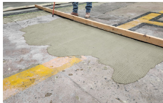
Elephant Armor® is applied in 3 panels to fill and level the repair area.
