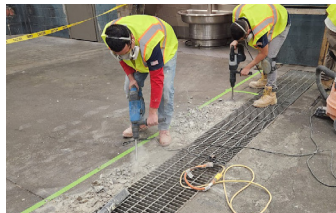
All loose unstable concrete is chipped away to provide a solid surface.
