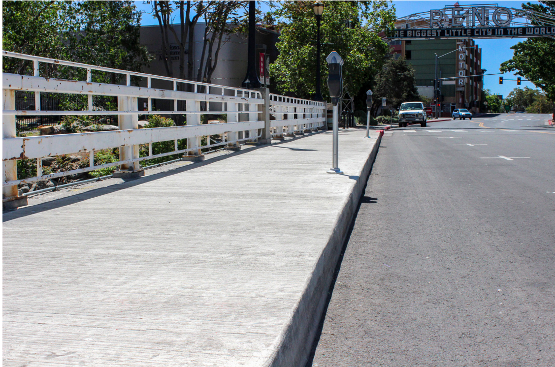
This repair was completed with a return to service in just 4 hours, saving the city weeks of time, money and significantly reducing the environmental impact and disruption of foot and vehicular traffic.
