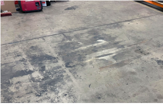
Damaged and unsightly warehouse floor panel prior to resurfacing.
