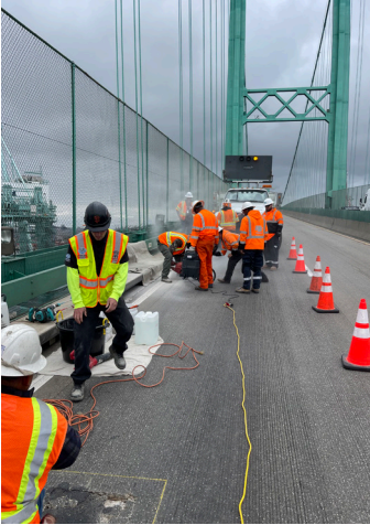
Photo showing a deteriorating asphalt filled pothole on a concrete bridge deck.
