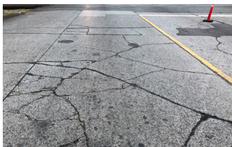
Distressed concrete roadway.
