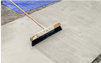
After GST Squeegee Trowel is used to smooth the surface, a broom finish is applied.
