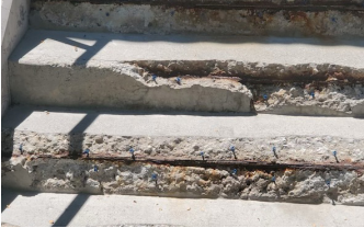
Concrete stairs degraded down to exposed steel.
