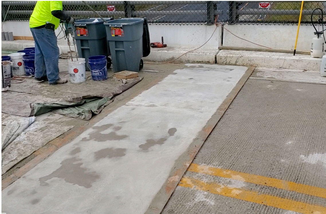
Bridge link construction completed in just 4 hours. Elephant Armor® was chosen due to its high compressive, flexural and tensile strength. Its fast setting properties allow for minimal shut down time and a quick return to service.
