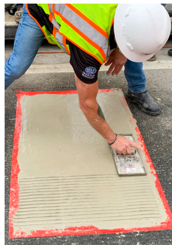
A tining trowel is then applied to the surface to match the existing bridge deck grooved surface.
