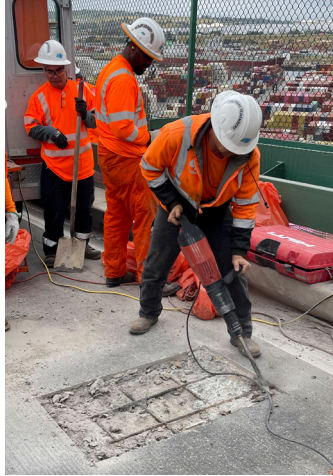
The damaged surface is removed and any loose material is cleaned away with a broom and a blower.
