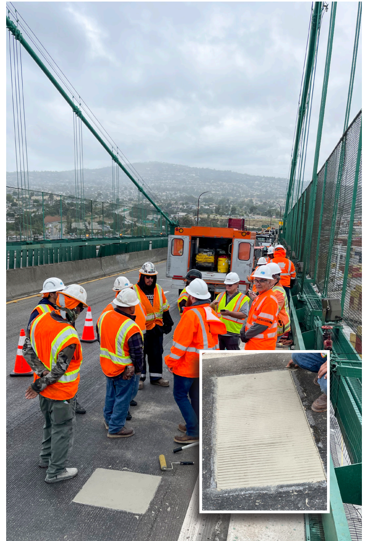
Elephant Armor's ease of use and quick set time, allowed the pothole to be permanently repaired with a minimum disruption to bridge traffic. This lane was back to service in less than 3 hours!
