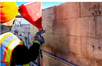
Surface Armor™ is sprayed on the degraded block wall after an initial application of Vetrofluid®.
