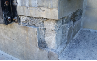
Extreme damage to loading dock.
