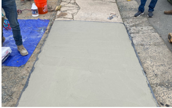
After cracks are prefilled, a 1/4" lift of Elephant Armor® is applied to the surface.
