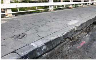
Badly cracked and spalled concrete sidewalk.
