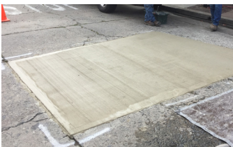
Repair completed in two hours and open to traffic in four hours.
