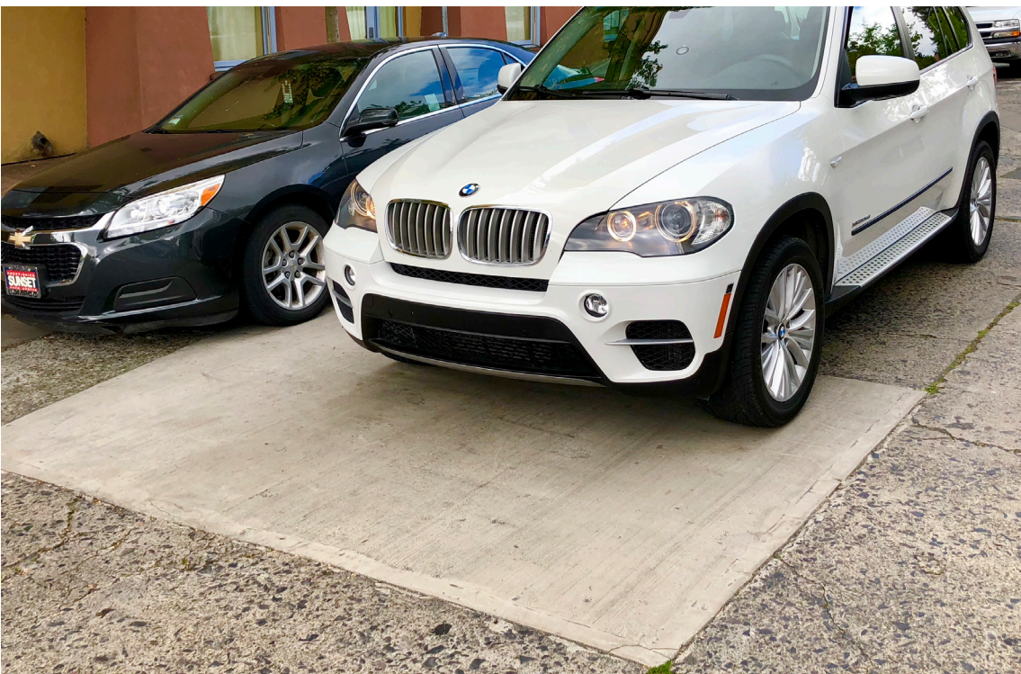
Repaired road panel 5 years after installation is still performing perfectly. With minimal environmental impact by significantly reducing the time of repair, a new lifecycle is achieved while also reducing repair costs by as much as 50%.
