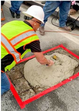
A GST Textured Roller is used to place and evenly spread out the high fiber mix design of Elephant Armor®.
