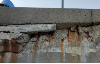
Broken and spalled seawall.
