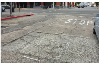
Failing road panel.
