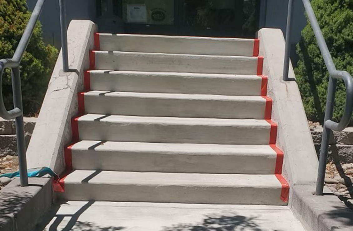
Severely weathered and broken stair treads made new, extending the lifecycle with Elephant Armor®. Repair completed by Morgan Construction, Reno, NV.
