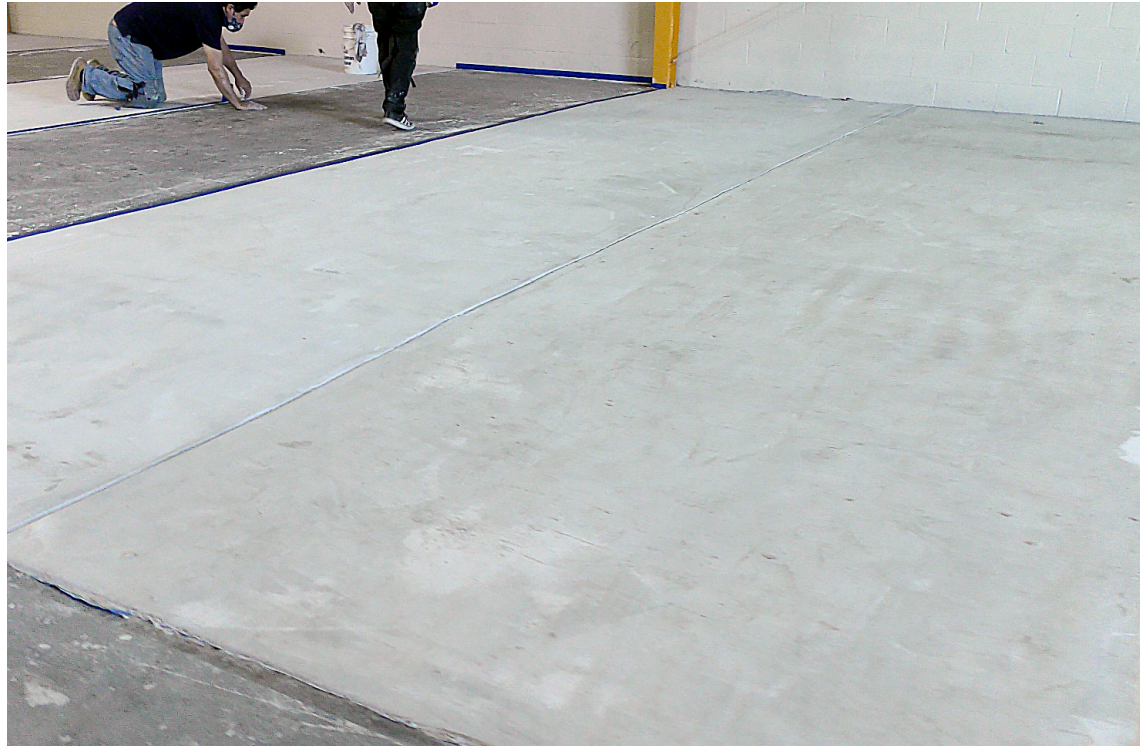
The installation was completed in sections allowing for uninterrupted use of the warehouse, saving 80% of the original remove and replace estimate.
