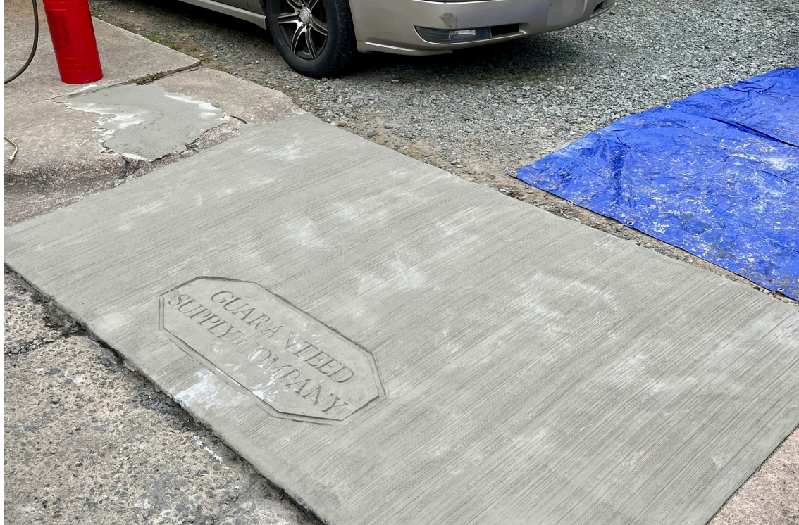
Finished repair stamped with Guaranteed Supply Company logo. Ecobeton®-USA VetroFluid® is applied as a last step after the Elephant Armor® repair has achieved a full cure.
