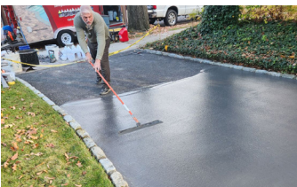
Driveway is given a new visual and service life with a final application of Ecobeton-USA® Vetrofluid®.
