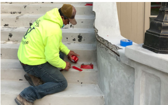
Severely broken and degraded wall cap.
