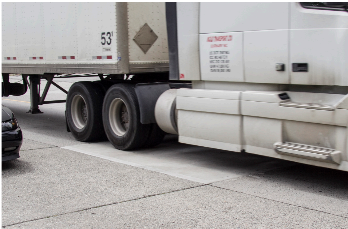
Roadway repaired for use in a matter of hours. Traffic volume in excess of 100 trucks per hour.
