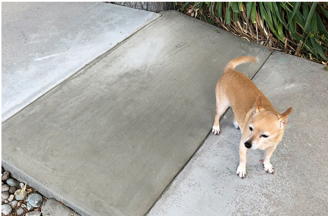
Trip and fall hazard was eliminated without having to remove the failing panel.
