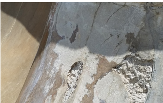
Damaged concrete surface unsafe for use.
