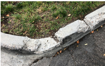
Severely damaged curb.
