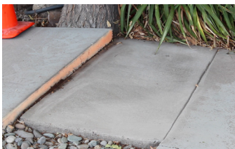
Extreme trip and fall hazard.
