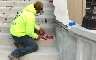
Severely broken and degraded wall cap.
