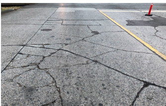
Distressed concrete roadway.
