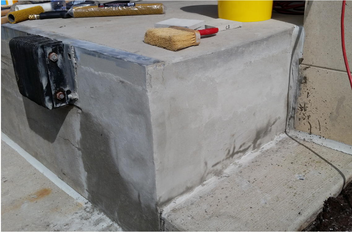
Damaged loading dock repaired without the need of forming and a lengthy interruption of service.
