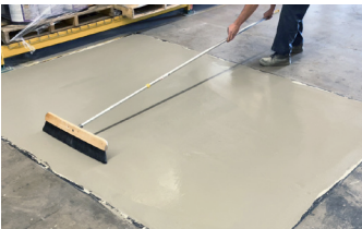
A no-slip broom finish is applied after the second coat of Surface Armor™.
