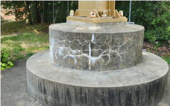
Ageing concrete showing cracking and calcium being released and formation of mold due to water retention.
