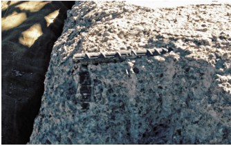
Spalled concrete with exposed rebar.
