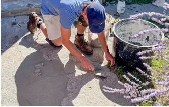
Elephant Armor® DOT used to fill all spalls, deep cracks and displacements. Forming not required.
