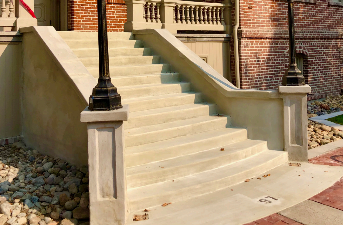
Damaged concrete stairs overlaid without deconstruction or forming, saving time, money and reducing the disruption of service.
