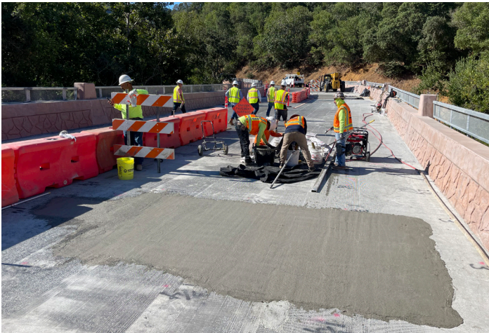
Areas with exposed rebar are filled and encapsulated with Elephant Armor® prior to final overlay application of Elephant Armor® DOT.
