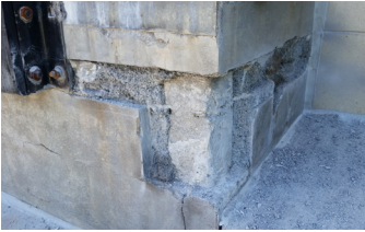
Extreme damage to loading dock.
