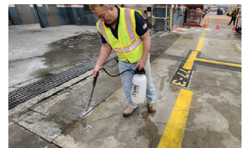
A coat of Ecobeton®-USA Vetrofluid® is applied to stabilize the existing concrete.
