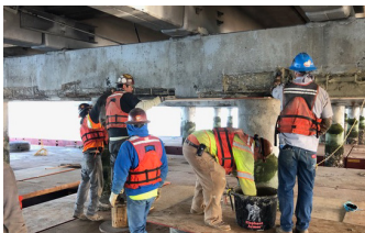
Applying a slurry primer coat over the repair area ahead of Elephant Armor® placement.
