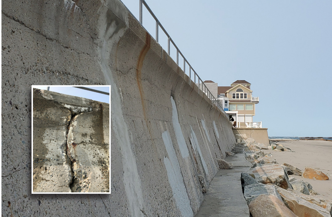
Severe fracturing of old seawall due to saltwater and weather exposure given new life using Elephant Armor® DOT.
