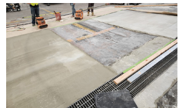
The last panel is ready to be filled and levelled with the two outside panels.
