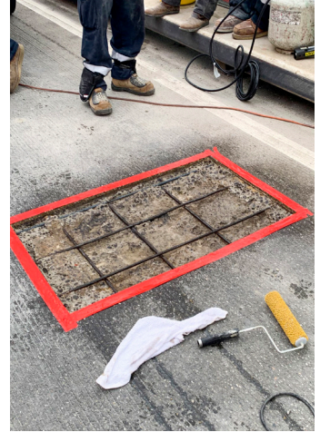
The clean and stable repair area is 'surface saturated dry' (SSD) prior to the placement of Elephant Armor®.
