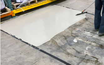
First coat of Surface Armor™ being applied with a GST Squeegee Trowel.
