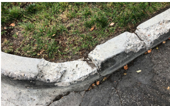
Severely damaged curb.
