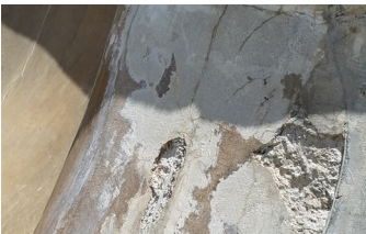
Damaged concrete surface unsafe for use.
