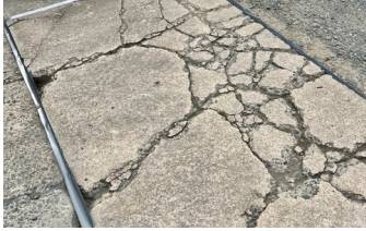
Severely degraded concrete panel ready for a 'fill and cap' application.
