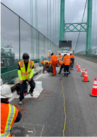
Photo showing a deteriorating asphalt filled pothole on a concrete bridge deck.
