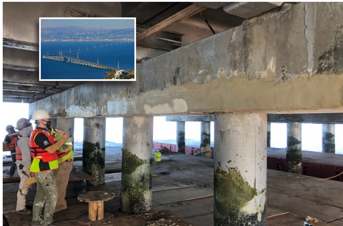
CalTrans using Elephant Armor® DOT on a 3 year project to bring the bridge back to its original specification without having to fully deconstruct and reconstruct the failing 1100 columns.
