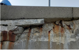
Broken and spalled seawall.
