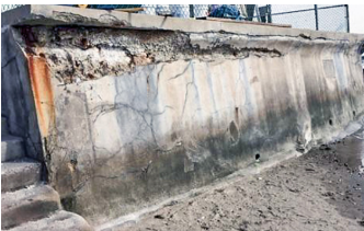
Severely degraded seawall.
